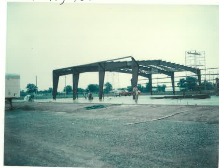
SERVICE GARAGE R/L
