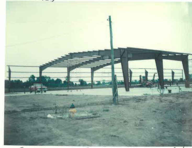
SERVICE GARAGE R/L
